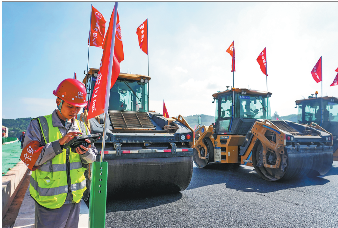
A technician monitors the operation of unmanned road rollers for a highway construction project in Mianyang, Sichuan province. XINHUA
