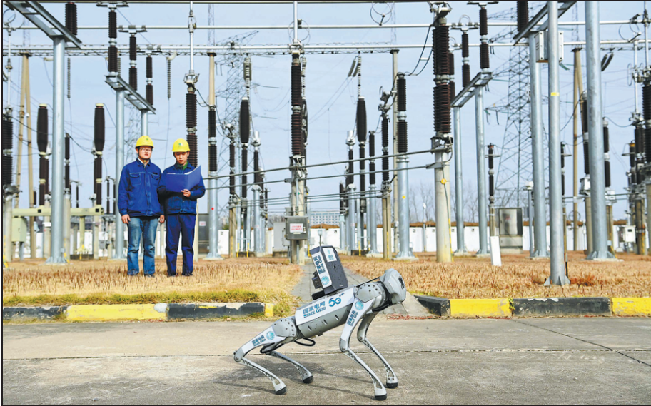
A smart robot and workers inspect power supply equipment at a 220-kilovolt substation in Chuzhou, Anhui province, on Jan 6. SONG WEIXING / FOR CHINA DAILY
