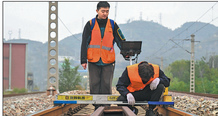
Two staff members from Taiyuan Track Works Section inspect rail lines in Shanxi province, aiming to rectify hidden defects and ensure the safe, orderly flow of passenger and freight trains during cold weather. SUN JIAHE / FOR CHINA DAILY
